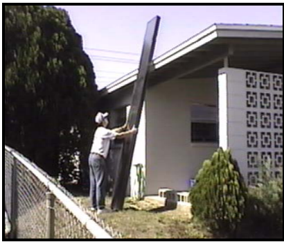
Protect Edge of Roof with a Tarp and Lean Collector Against Roof
