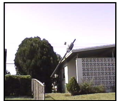
Move Up the Roof as you Pull the Collector Up a Foot or so at a Time.
